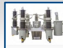
Pole-mounted Capacitor Banks
